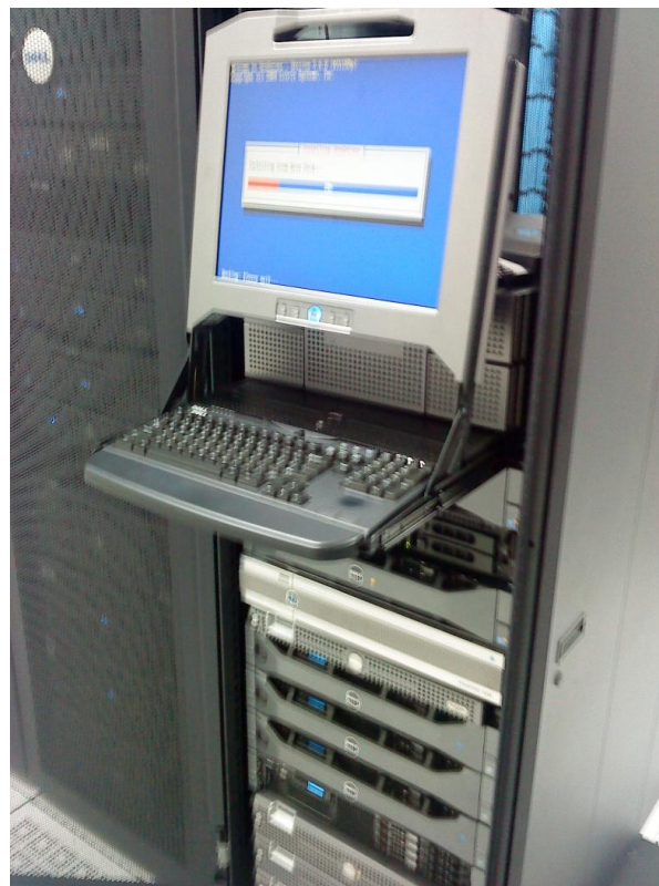
Figura 3.1 Rack de Servidores Dell Poweredge R710.
